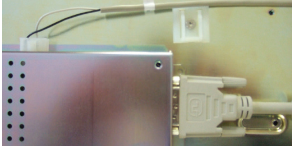
FIGURE 24 VIDEO AND POWER CONNECTIONS CONNECTED TO LCD
