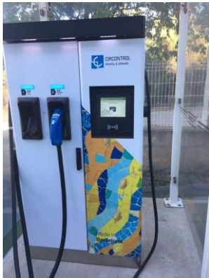
EV charging stations (Spain)
